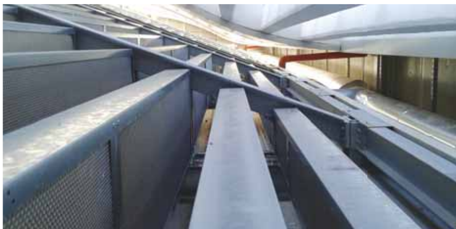
SA/LF acoustic baffles
