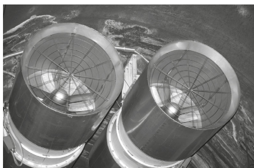
MCPA attenuators for tunnel
